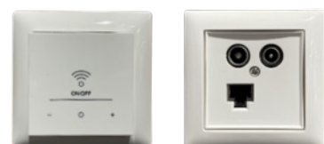
WLAN ACCESS-POINT TV/RADIO/LAN-ANSCHLUSS
